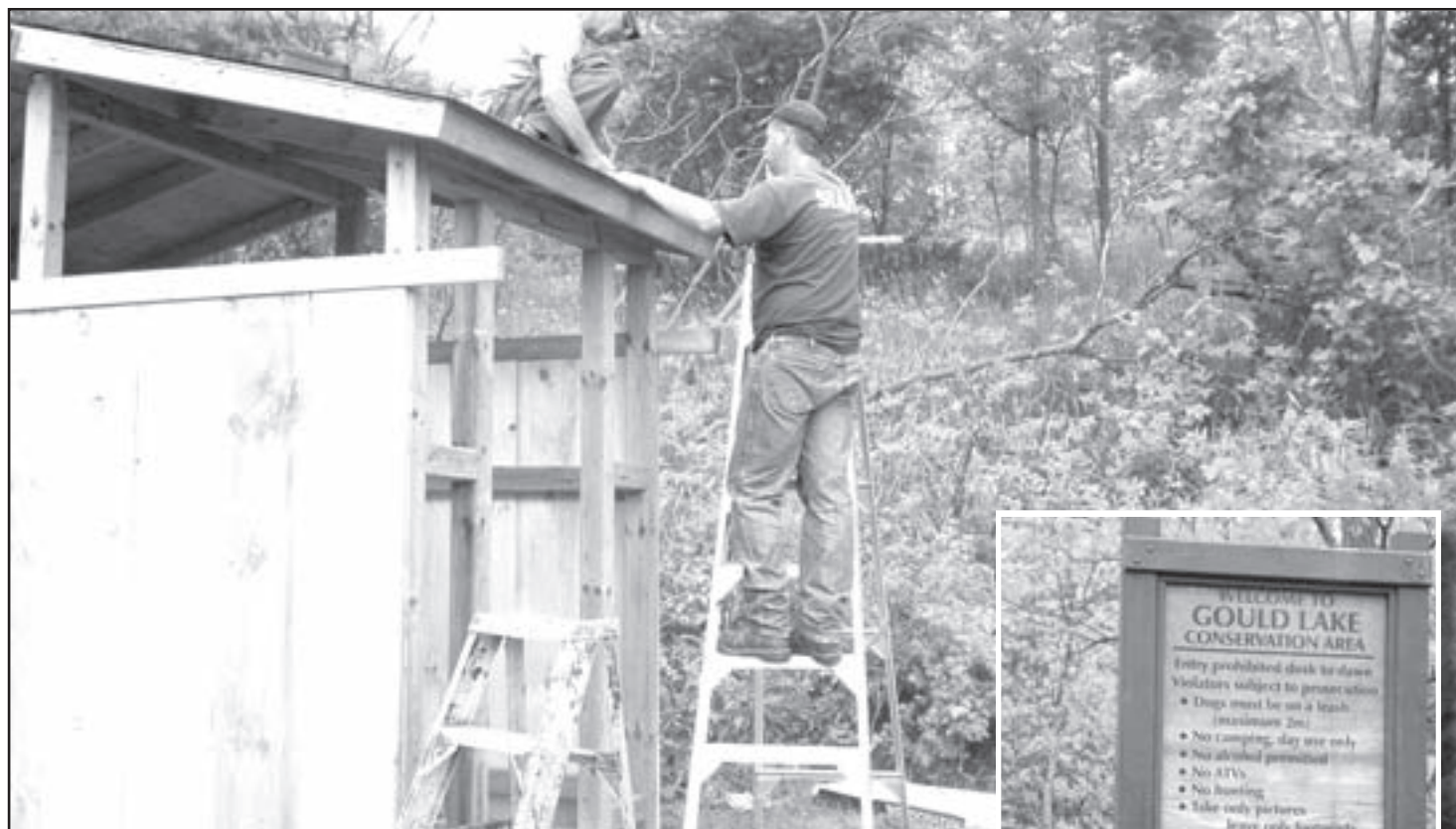
Ian Brown and Mike Ignas put the finishing touches on the roof of the new privies at Gould Lake Conservation Area.
